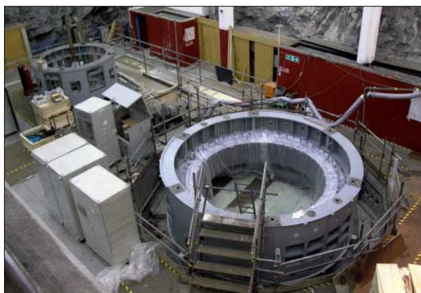
Shot of the refurbishment at Ceannacroc (20 MW), by Fort Augustus. It was accredited for ROCs in April 2003.
