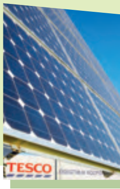
Solar panels at one of our stores in Hungary
