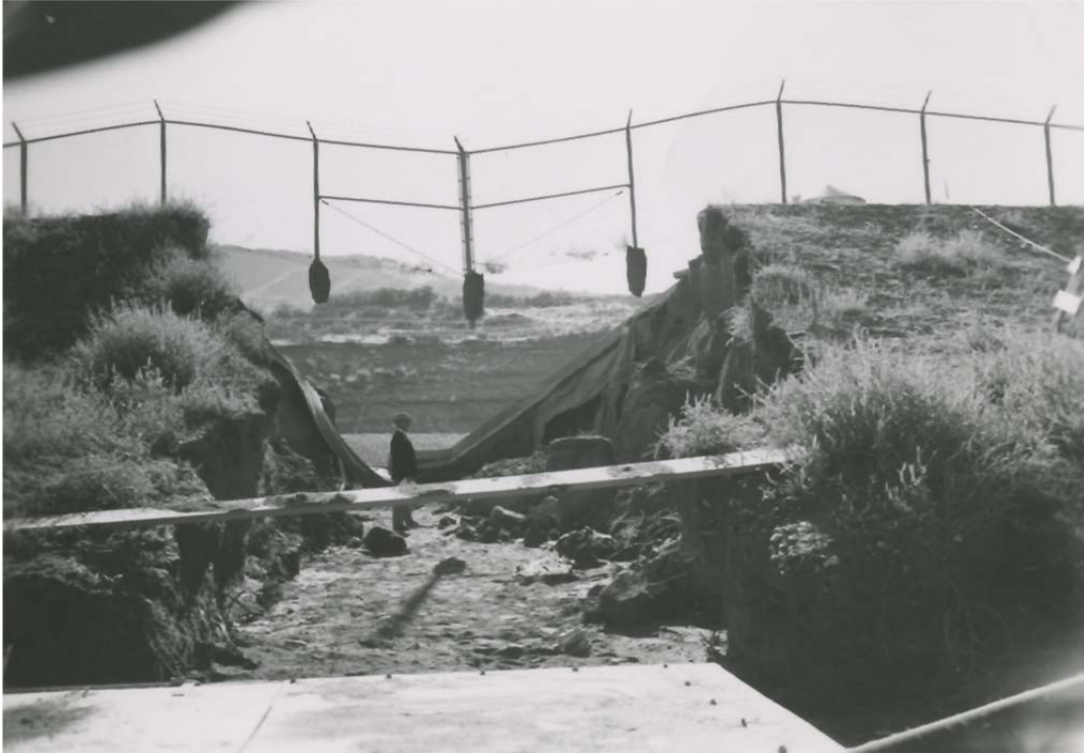
Close up of breach, Reservoir No.1 Dam Source: Earl Bud Bay, Reclamation, September 25, 1961
