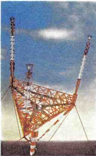
RCA designs and builds the equipment that transmits the TV signals.
