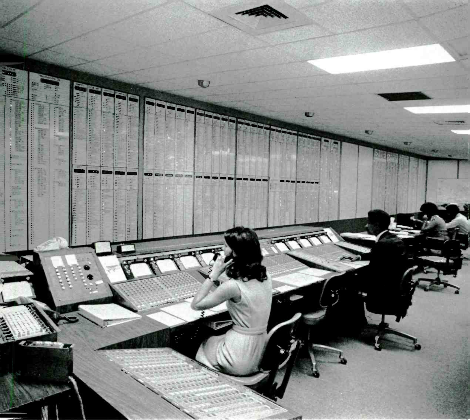
At the Network Management Center on East 38th Street, New York City, consoles and display boards help personnel monitor and control the operation of the downstate New York network. The Center is jointly operated by New York Telephone and AT&T Long Lines.
