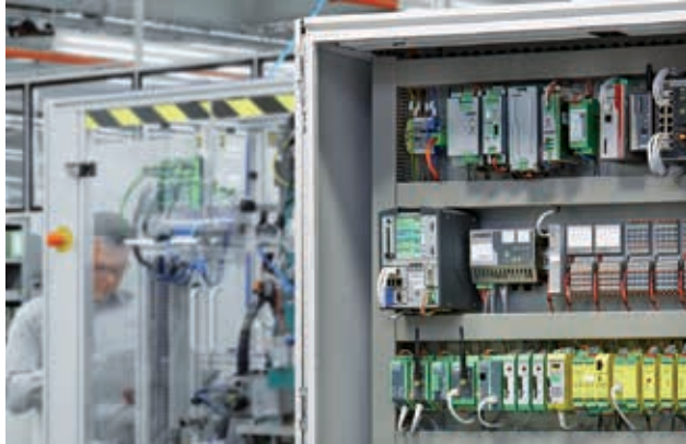
Figure 54: Machine control cabinet with signal and data connectors – source: Phoenix Contact
