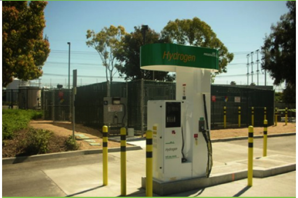
Photograph of the state-of-the-art hydrogen fueling station with fueling at 5,000 and 10,000 psi according to the latest SAE protocols for rapid 3-minute complete tank refueling.
